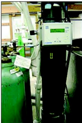
Water monitoring system and oxygenation tanks
