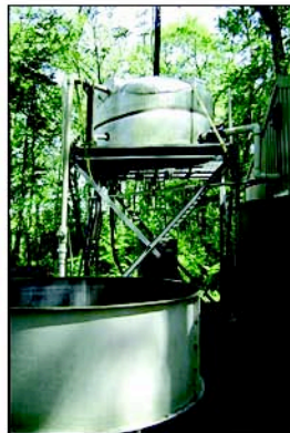
1,200 gallon elevated water tank
