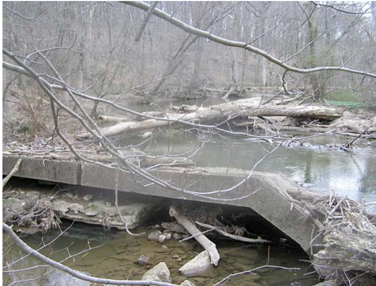
Figure 4.27. Slumping concrete at the race entrance of the former Yeatman’s Mill Dam
