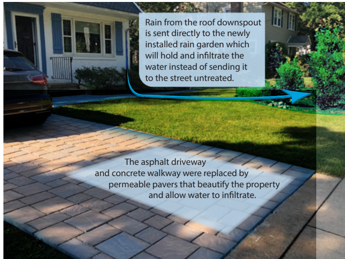
Permeable paver retrofit and rain garden installation in the city of Newark.
